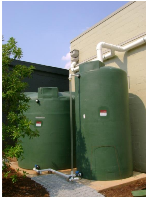
Rain Collection Tanks at Kendeda Center
